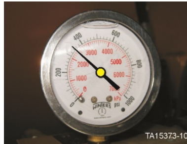
Figure 31. Pressure gauge with correct flow and pressure small flicker at about 350 psi (24 bar)
