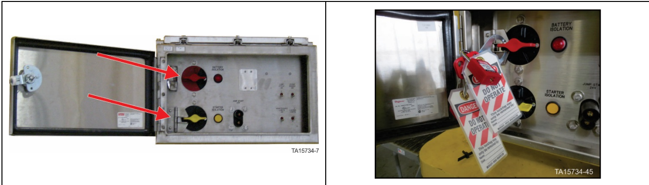
Figure 14. Battery Isolation Box – Battery isolation switch in OFF position with locks in place
