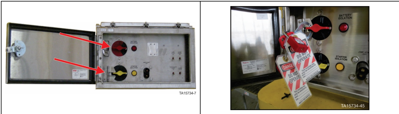
Figure 21. Battery Isolation Box – Battery isolation switch in OFF position with locks in place
