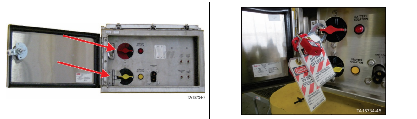
Figure 47. Battery Isolation Box – Battery isolation switch in OFF position with locks in place
