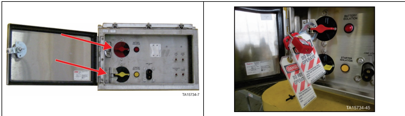
Figure 70. Battery Isolation Box – Battery isolation switch in OFF position with locks in place
